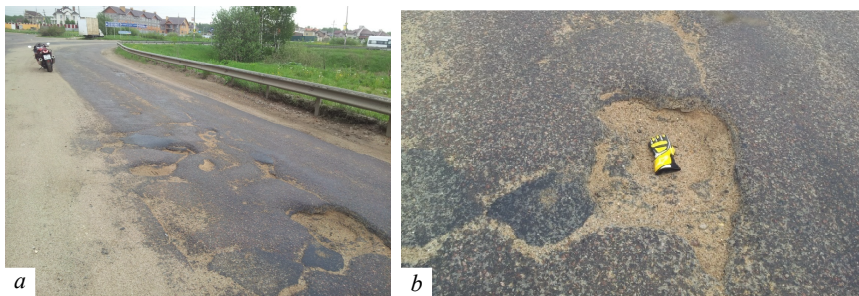
Fig. 1. Photos of potholes in a paving: a ) a general view of a road situation; b ) a glove of the driver of the motorcycle in a hollow
